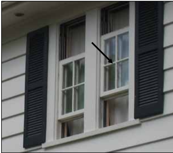
Example of muntins on a pair of historic wood windows. Photo courtesy of Patty Spencer
