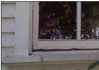
Example of a window that will not close completely because it is racked
